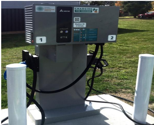
Charging Station Harcourt
